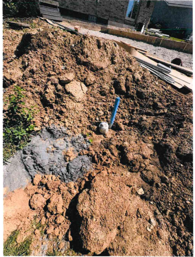
Disturbance around septic tank and clean out.
